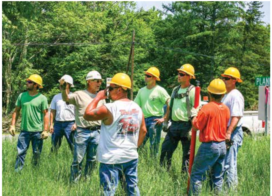
GAME PLAN: Claverack REC’s Wysox Crew Chief Lindsay Chamberlain, third from left, discusses line repairs with Tri-County REC work crews after a tornado ripped through parts of Tri-County’s service territory in May 2011. Through their C&T Enterprises partnership, Claverack and Tri-County, along with their affiliated electric utilities, Citizens’ Electric of Lewisburg and Wellsboro Electric, have the ability to share personnel resources during outages.
