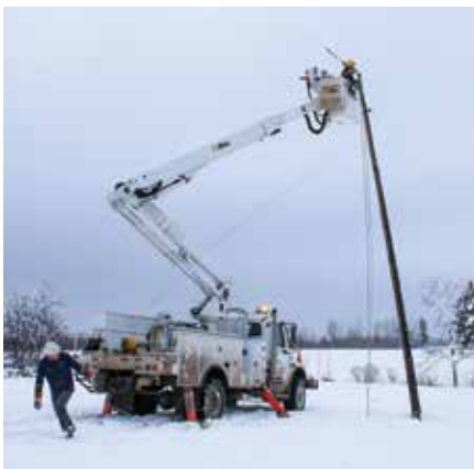
STORM SUPPORT: During times of major storm damage, Claverack can count on a network of cooperatives from Pennsylvania and New Jersey to provide mutual restoration assistance. Above, Claverack and Central Electric Cooperative crews work to restore power after a January 2021 snowstorm caused widespread outages across Claverack’s service territory.
