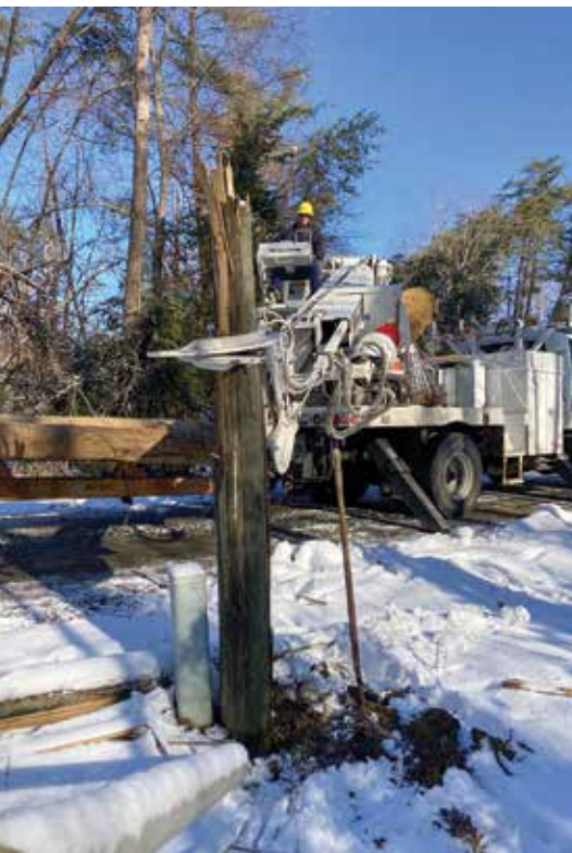
SNAPPED: Claverack’s Tunkhannock District crew chief, Brandon Griffiths, removes the splintered remains of a utility pole from a Northern Neck Electric Cooperative member’s property. The Virginia cooperative reported that 50 poles were broken during the Jan. 3. snowstorm.
