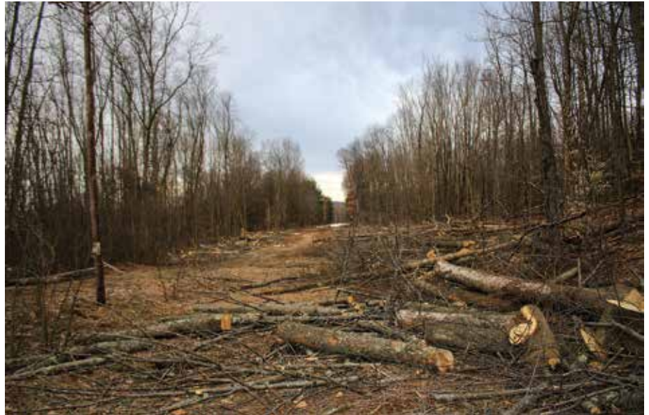
DANGER DOWN: The fallen remains of ash danger trees litter the sides of a Claverack right of way in Bradford County after a contract tree crew cut them down last year to prevent them from falling onto co-op lines.
