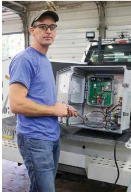
GETTING READY: Claverack electronic technician Larry Beebe prepares networking equipment for installation as part of the co-op's advanced metering infrastructure (AMI) project that began in October. The cooperative plans to replace all of the existing meters on its system over the next two years as part of the AMI project. The new wireless metering system will offer real-time meter-reading and outage-reporting capabilities.
