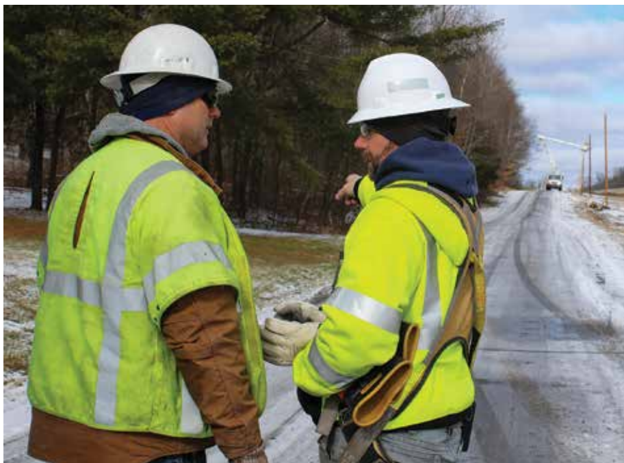
LINE RELOCATION: Montrose Crew Chief Allen Scott, left, and Manager of Field Operations Bucky Camburn discuss details of a line relocation project near Lawton in Bradford County in January. Scott and Camburn began working for the co-op in 1998 and 1997, respectively.
