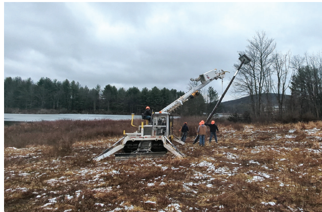
HABITAT RESTORATION: Lineworkers from Claverack Rural Electric Cooperative's Wysox District install osprey habitats on State Game Land 250 in partnership with the Pennsylvania Game Commission.
