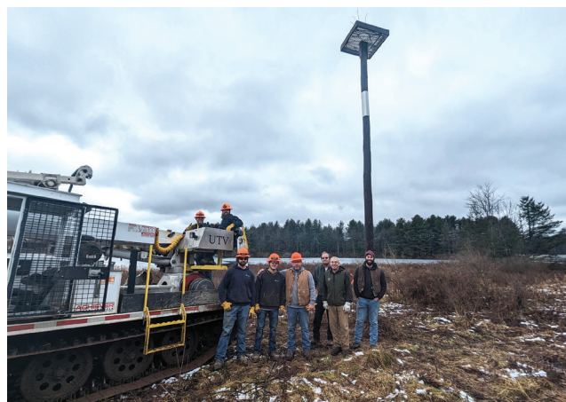
COMMUNITY PARTNERS: Members of the Pennsylvania Game Commission (PGC) join lineworkers from Claverack Rural Electric Cooperative's (REC) Wysox District following the installation of a new osprey habitat. Shown, from left, are: Claverack REC lineworkers Leonard Fowler, Jeremiah Lund, Nate Hoke, Adam Rosenberger, and Rich Herman and PGC employees Mike Finan, Darren Pettyjohn, and Evan Delp.
