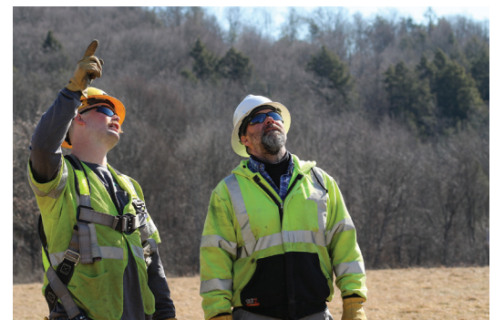
UPKEEPING LINES: Above, Claverack Rural Electric Cooperative (REC) lineworkers prepare to set new utility poles. Below, from left, Isaac Dibble, apprentice lineman, and John Camburn, manager of field operations, inspect cooperative power lines.
